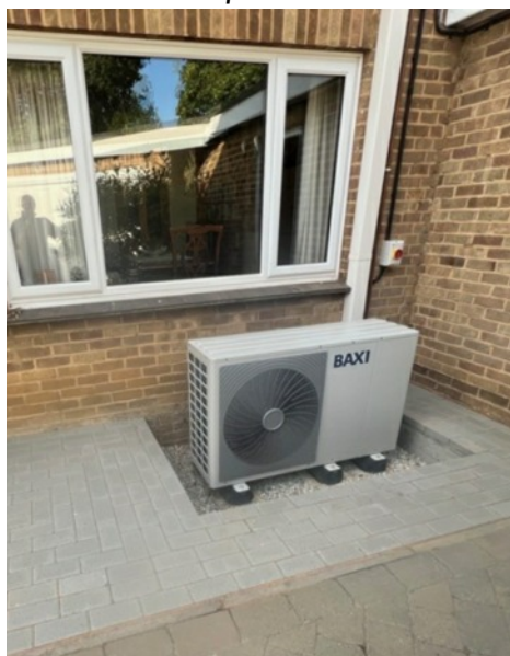
The heat pump outside the back door
