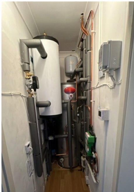
The equipment installed in the airing cupboard
