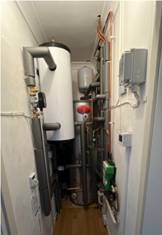
The equipment installed in the airing cupboard
